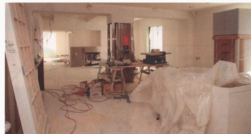
Pella™ windows and Joanne Hudson cabinetry await installation in the contemporary flat.
